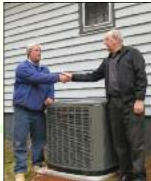
When his 20-year old heat pump failed, HEMC member Dean Dyer took advantage of the How$mart program and had a new, high-efficiency Trane 15-SEER heat pump installed by Peak Performance Heating & Air of Cleveland.
